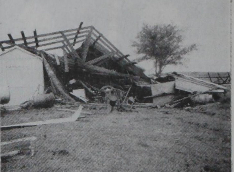
STORM DAMAGE: Thursday night, the area was not under tornado warning or alert, but a small tornado apparently moved across the lower part of Hemphill County. Up to 4" of rain was reported in some areas. This barn, built in the late 1800's is on the Helton Ranch, 7 miles north of Allison. Other barns were moved from their foundations and destroyed. The Truck was west of the barn with a house between.
