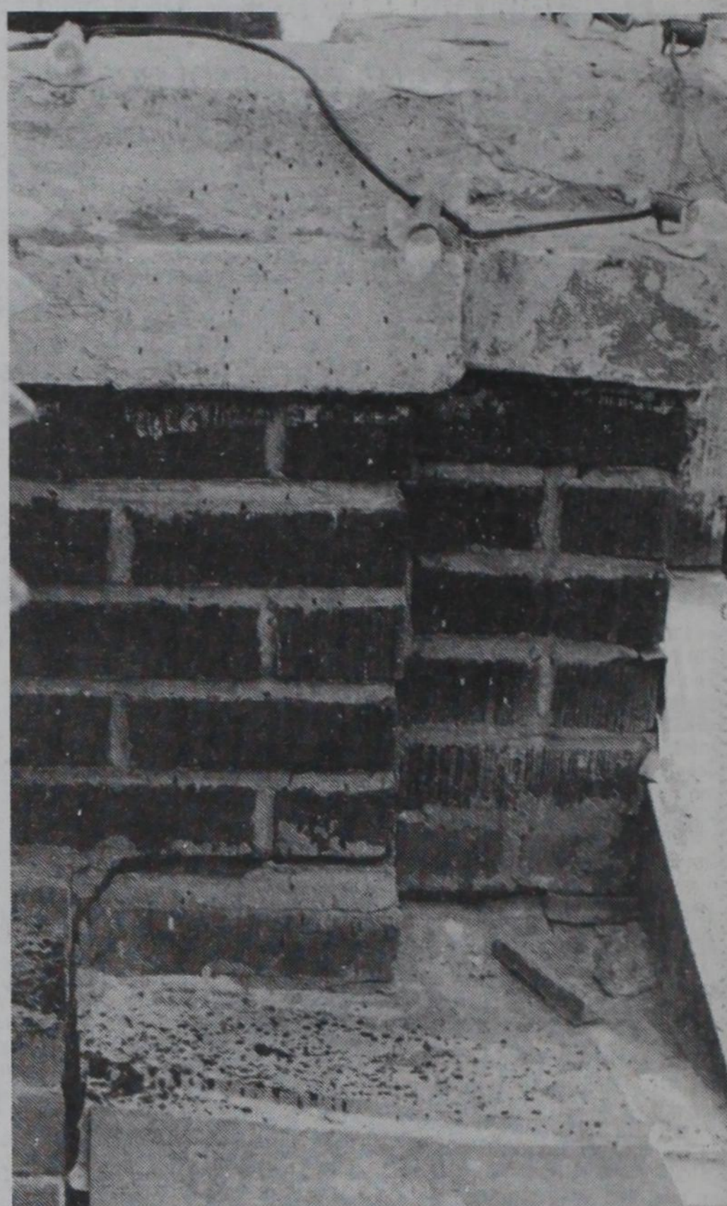
Water stands in basement storage area in courthouse basement
