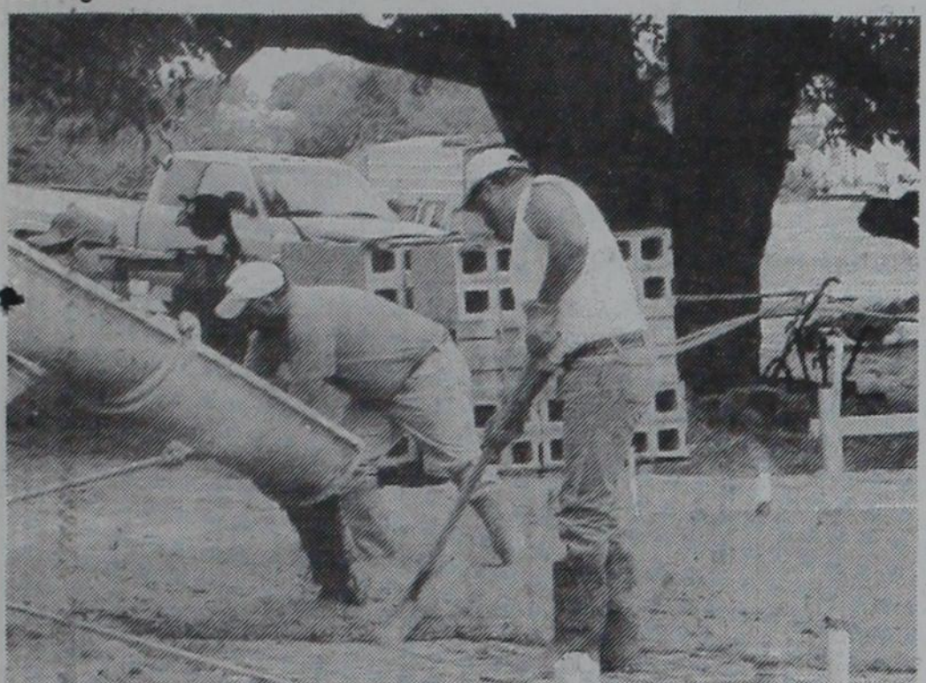
CEMENT ARRIVES: Canadian Supply and Redi Mix arrived at Mobeetie Thursday and the slab for the restrooms was poured. Shown here are (l. to r.) Martin Perez, Lous Perez and Armando Mederano.
