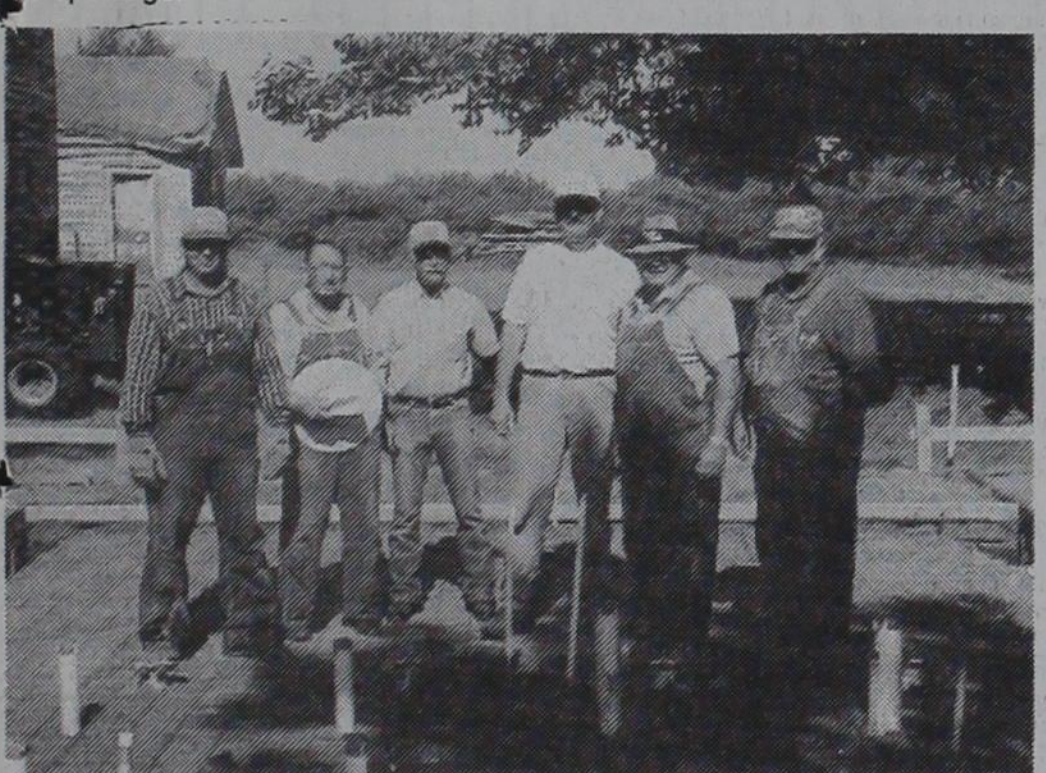
VOLUNTEERS: Several volunteers were on hand to help with the pouring of the slab for the restrooms at the Old Jail Museum. Pictured here are (l. to r.) Bill Finsterwald, Don Burke, Geoff Caldwell, Jay Godwin of Canadian, Nathan Lancaster of Pampa and Bill Hagerman of Pampa.
