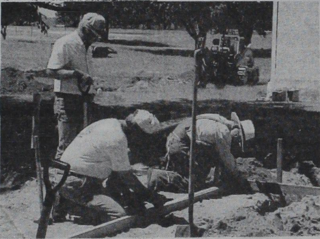
FINISHING TOUCHES: All the corners have to be filled in just right before the slab can be poured. The concrete was to have arrived Wednesday, May 30. The bathrooms are to be finished in time for the Bluegrass Festival on July 27 thru 29, 2001. Pictured (l. to r.) Geoff Caldwell, Jay Godwin and Arthur Don Burke. Bill Finsterwald was also helping.
