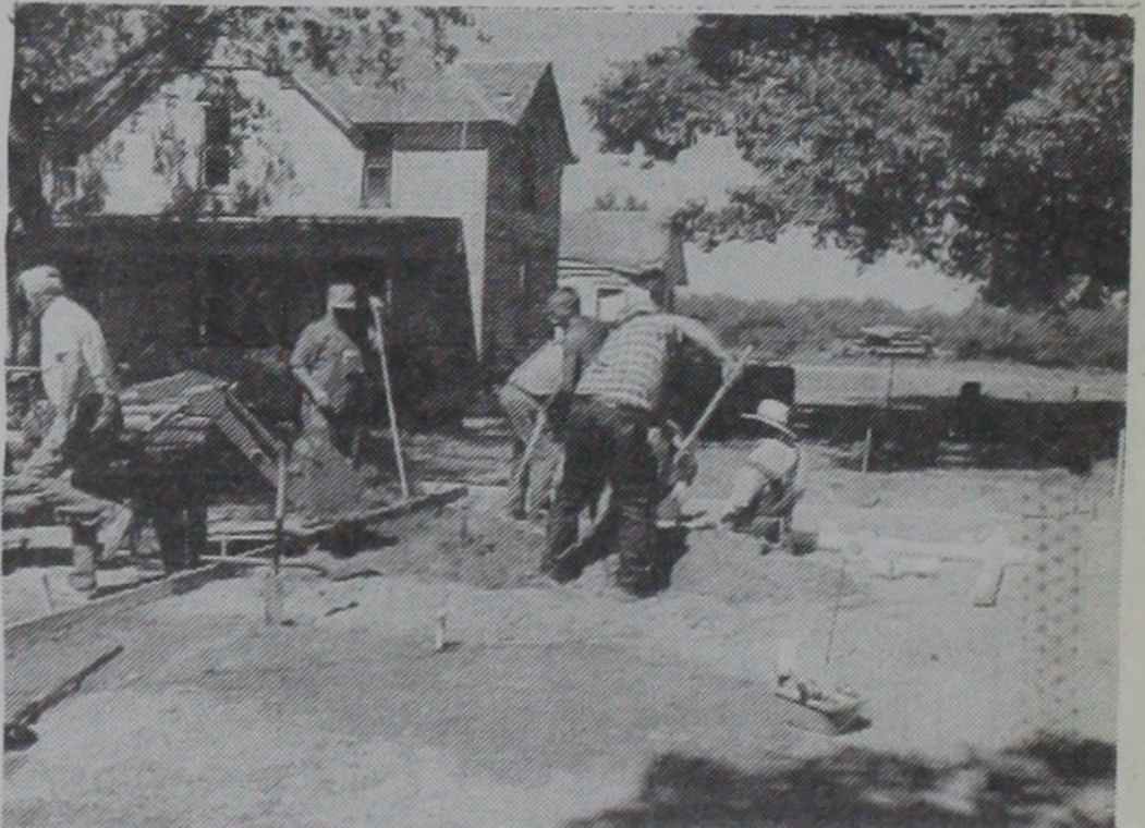
WORK BEGINS: Volunteers began working on the slab for the Old Mobeetie Jail and Campground restrooms on Wednesday, May 23. Pictured working here are: (l. to r.) Bill Elliott, Bill Hagerman, Larry Jennings, Bill Corcoran, Bob Meller and Don Burke. —Photo by Melba Corcoran
