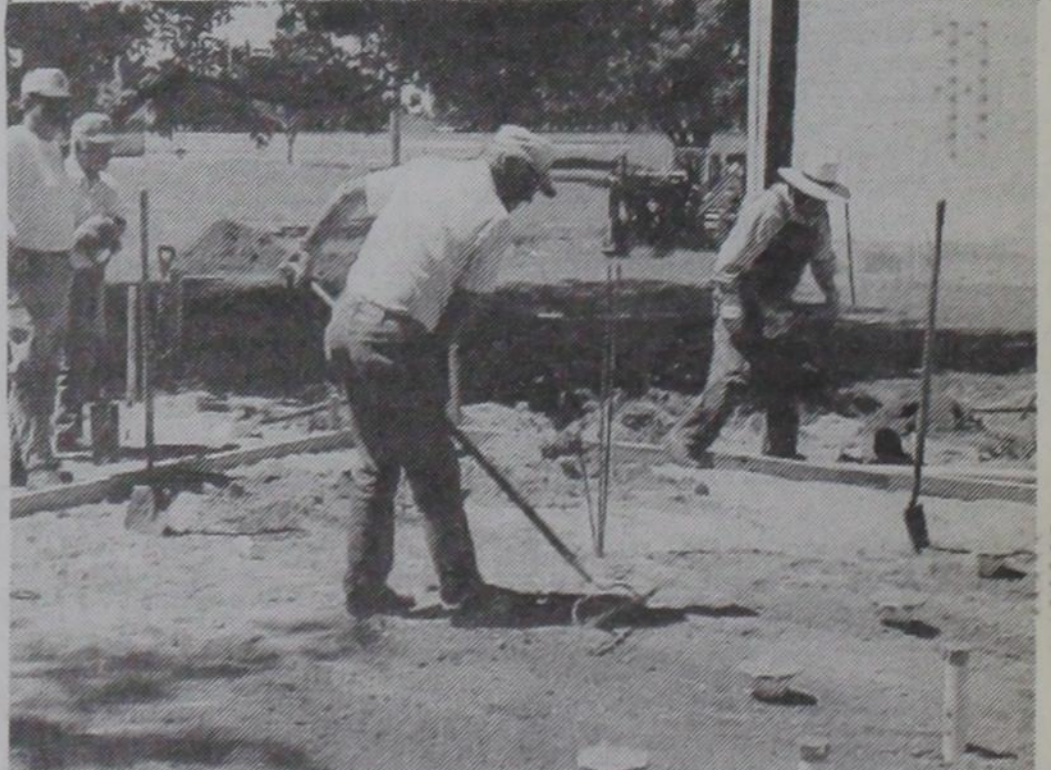
LEVELLING BEGINS: With the plumbing in place, the leveling begins in preparation for the pouring of the slab. Pictured are (l. to r.) Jay Godwin, Geoff Caldwell, Bill Elliott and Arthur Don Burke. —Photo by Melba Corcoran
