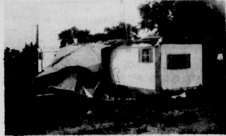
DAMAGED STURDAY EVENING: The trailer home of Mr. and Mrs. Harold L. Jones had the roof removed about 10:30 Saturday Evening. The trailer is located northwest of Wheeler, just outside of the city limits. The sound was similar to that of a jet passing over at the time of the damage. The Jones had been visiting her parents, Mr. and Mrs. Marvin Underwood until about 10 when they went home to go to bed. The inside of the trailer received some water damage. A few limbs broken around the Underwood home was the only other damage.
