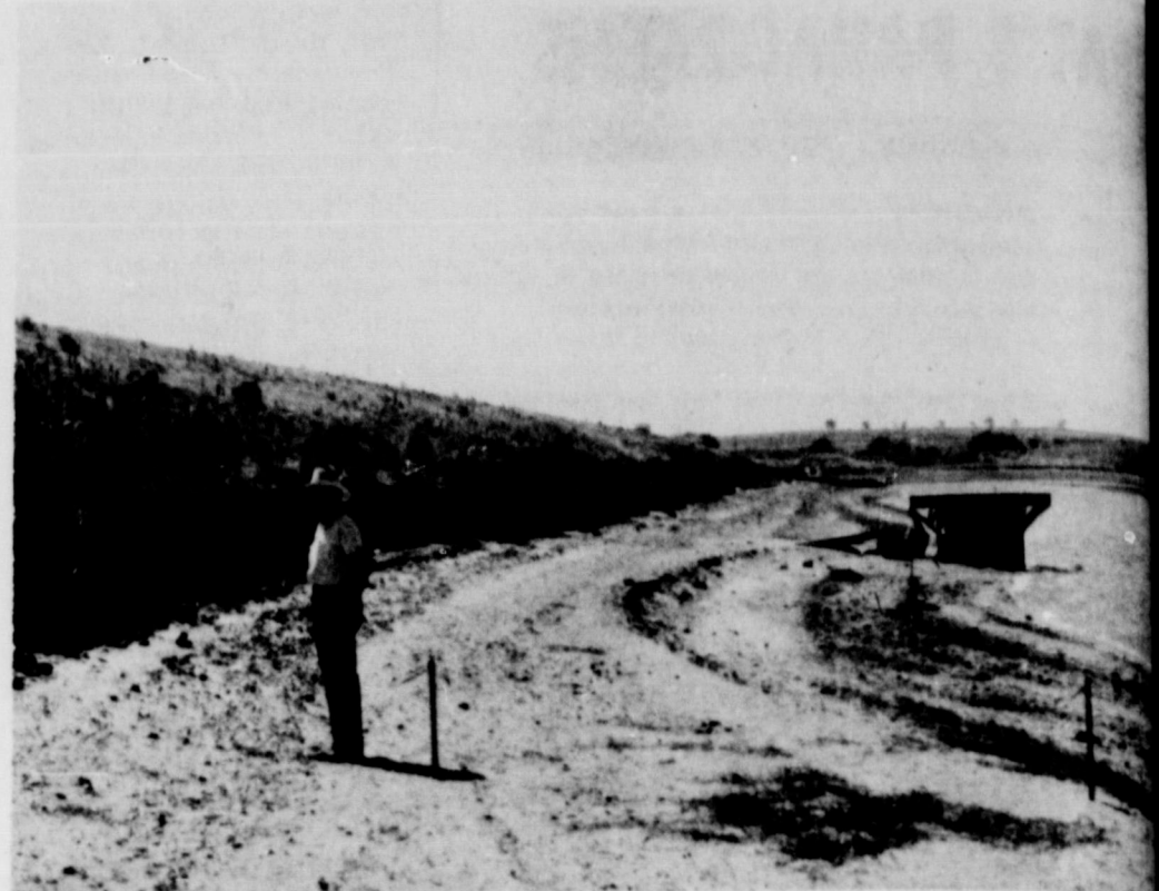
CONSERVATION NEWS: The front of this dam in the northern part of Wheeler County faced to the south. The prevailing wind caused more than usual wave action against the dam. The constant beat of the waves eventually washed away a large portion of the dam. The water had to be lowered and large rock was placed all along the front of the dam to protect it against wave erosion.
