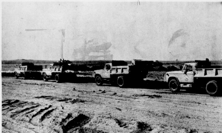
NEW SITE ---Texas Highway Department equipment moves in on a plot of land on the south side of U. S. Highway 84 on the outskirts of Muleshoe and have begun preparing the ground for a new department facility to be constructed. Work on the buildings is expected to begin in two weeks.
