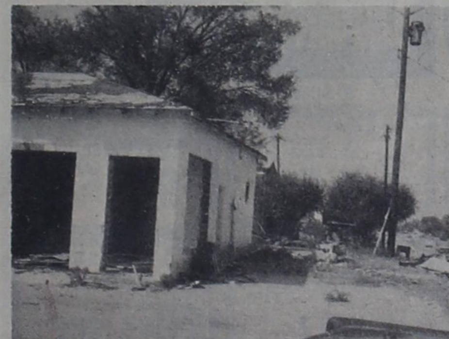
MAKING WAY FOR PROGRESS: This property at the intersection of highways 83 and 152 in Wheeler is being cleared for the construction of a convenience store. The service station and machine shop was operated for a number of years by the late Fred Farmer. The front part was used by L. & F. Repair when they started in business 10 years ago. The front part was last used for a body shop by Pete Burton. The razing of the building began this week.
