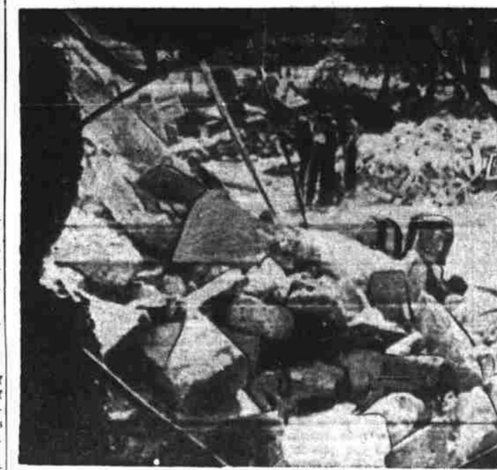
Framed by a hole blasted by a bomb in a wall, these workmen here are shown clearing debris in the center of Warsaw. (Associated Press Cablephoto from London.)
