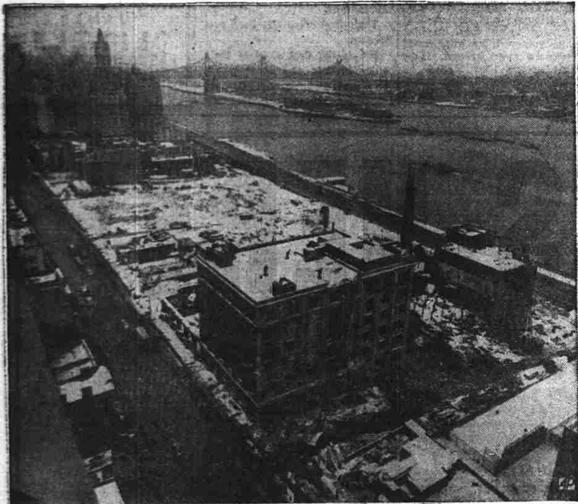
UN HOME SITE —Two buildings (foreground) remain to be razed at site of new United Nations home on New York's East River. Scene is looking north from 42nd St. on 1st Ave.
