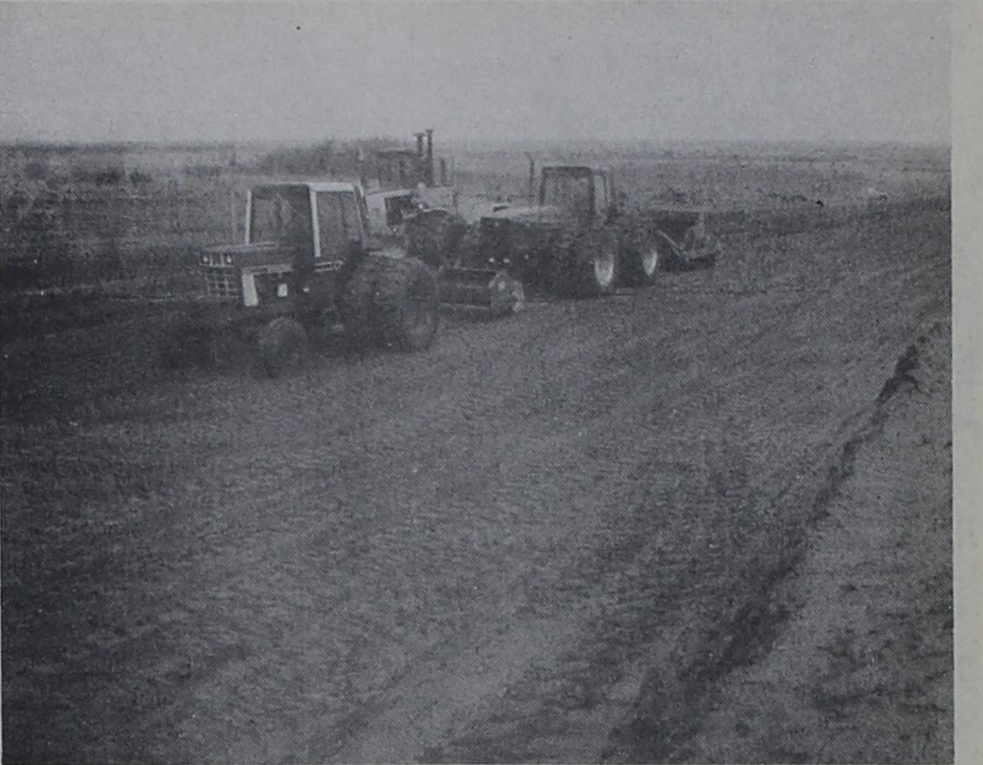
AIRPORT: Dirtwork work has begun at the site of the new Wheeler airport. The area had to be fenced before the farm tractors were brought in to level the 3500 foot strip. Local individuals have donated farm equipment and manhours for this project. This picture was
