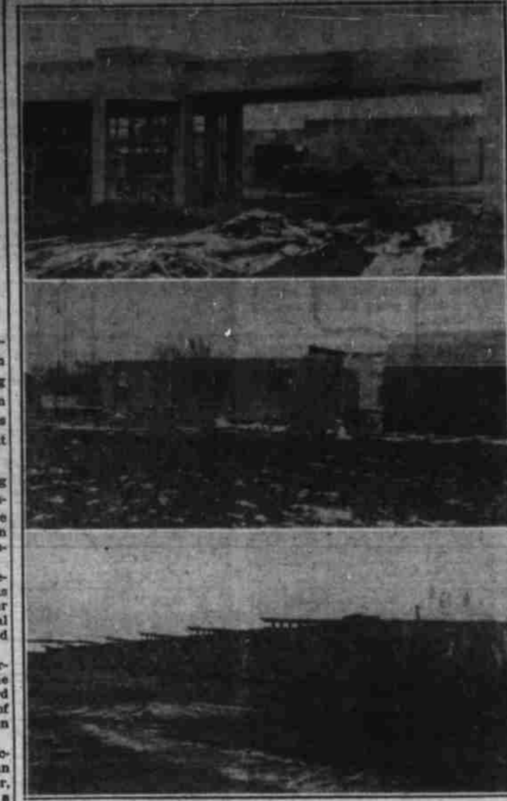
These are samples of increasing construction going on in Big Spring in the early months of 1938. Top view is that of the Standard Oil company new $7,500 station being raised at the corner of E. 3rd and Nolan streets. Center is the $3,500 home being built by Edmond Nottelme at 1504 Johnson street. Below is the recently completed $12,000 addition to the compress on N. W. 3rd and N. Gregg streets. The top of the original compress warehouse is in the distance.
