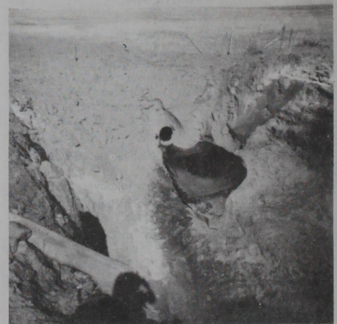
PIPELINE EXPLOSION: Wheeler and Mobeetie Fire Departments were called to the scene of a pipeline explosion early Monday morning. A 26" pipeline belonging to Natural Gas Pipeline Co. exploded, causing a hole 20' deep, 15' wide and 60' long in the middle of Gray Co. Rd. 29, just across Wheeler County line and 1/2 mile north of Highway 152. No injuries were reported. The Wheeler Ambulance Service was also on the scene.
