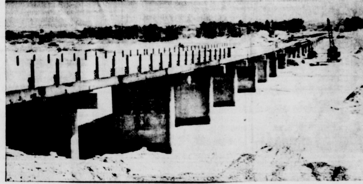
AUGUST COMPLETION DATE: T. A. Mussett, foreman of the Strain Brothers Construction Company crew working on the new bridge across the Red River, has changed the completion date from July 1st until August 1st. Mr. Mussett contributes the delay to bad weather.
