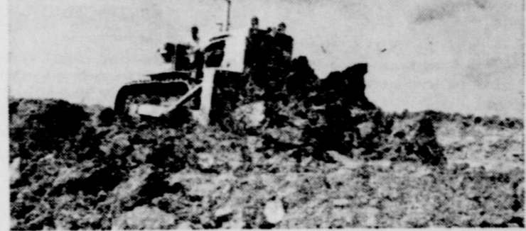
BEAR for work is this new International TD-25 crawler tractor, here moving huge load of earth on runway extension project at Chicago's jet-age O'Hare International airport.
