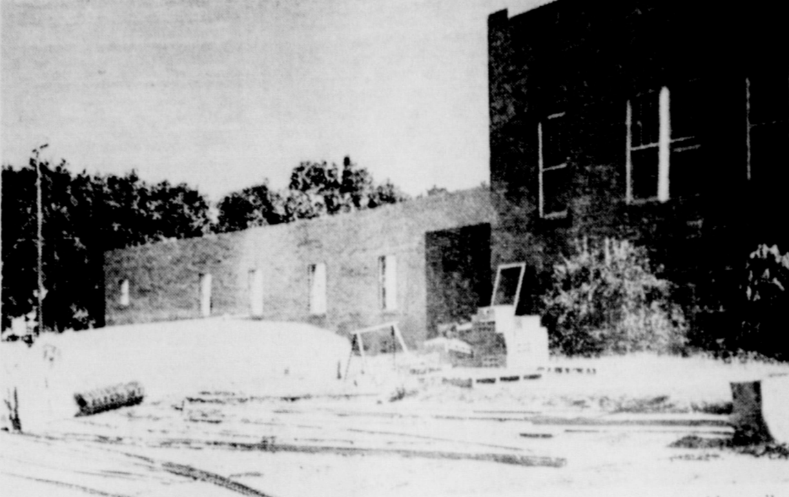
BAPTIST PROGRESSING ON BUILDING: All of the brick is laid, the outside walls are complete, the inside tile is laid, the partitions are all erected, the plumbing is roughed in and the sheeting for the roof will be complete this week. Construction foreman, L. D. Atchison indicated that workmen will have the entire roof and exterior completed by the end of the week. The Baptists hope to have the new education building completed entirely sometime in October.
