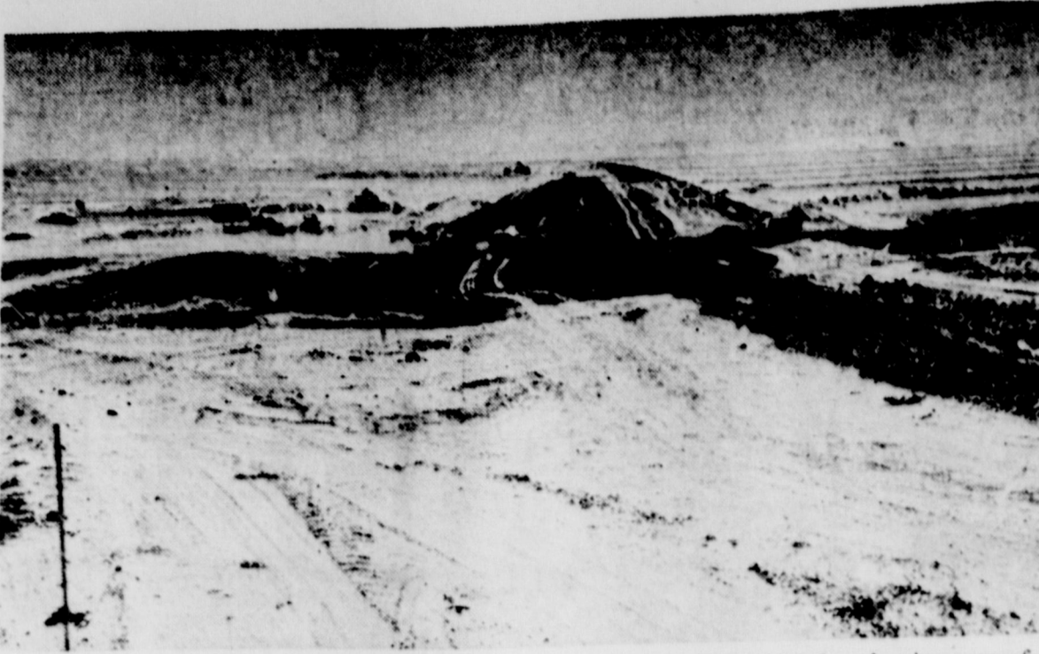
SITE 18: Work on site 18, pictured above, and site 19 was halted Wednesday because of the 4 to 5 inch rain Tuesday night. However, work is progressing rapidly and both dams will probably be completed by September. The above photo is looking West on site 18, which will have a 36 acre sediment pool; 817 acre feet of flood storage; and the dam will be 34 feet high. It will have 51 cubic yards of concrete, 1,926 lbs. of reinforcing steel, 216 feet of concrete pipe and 6,632 feet of facing. The DePauw Construction Co. of Amarillo is the contractor
