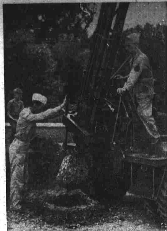
SUBJECT IS BORING —Spade and shovel methods of digging tank traps and other defense holes appear doomed, now that an earth borer such as this from the Buda plant at Harvey, Ill., has been introduced. It is designed for use in warfare also to facilitate the laying of land mines. The men are non-commissioned U. S. army officers testing operation.
