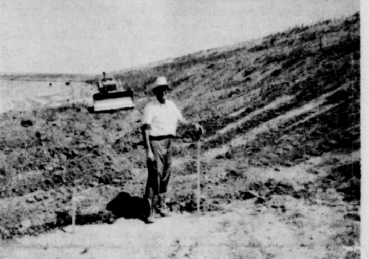
FINSTERWALD DAM: Repair work on the Finsterwald dam, a watershed structure of the Washita watershed, has begun. Wave action on the front side of the dam has cut into the structure. The washed out area will be shaped and a rock rip rap will be placed on the face of the dam to prevent damage in the future. O. W. Sweat of Spur is the inspector for the job.
