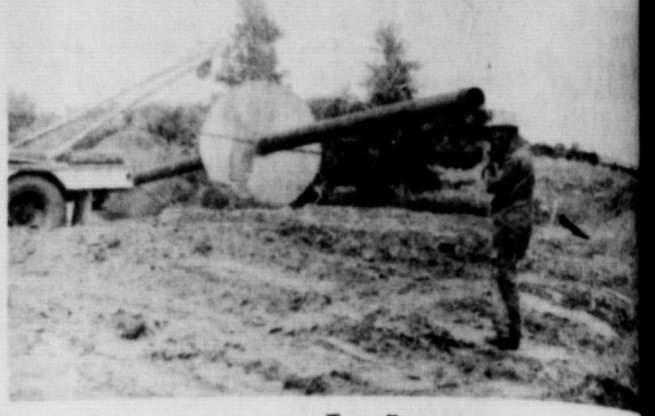
In this picture you see Tom Puryear assisting construction contractor install a pipe in his farm pond. Notice the round disc type objects welded onto the pipe. These are anti seep collars that prevent water from finding its way down the outside of the pipe and eventually washing out the dam. This pond will furnish sufficient water for livestock that formerly did not have adequate water. It also cause livestock to graze the pasture more uniformly. Design and layout of the pond was by Soil Conservation Technicians that assist the Wheeler County Soil and Water Conservation District.
