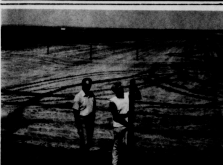
Beef Cattle Co., Inc. is constructing a new 15,000 head feedlot to serve Wheeler County and the Eastern Panhandle. The construction is estimated to cost about $450,000 and is located three miles Northwest of Wheeler on Highway 152. This will be a fully automated lot equip to handle all classes of cattle.
