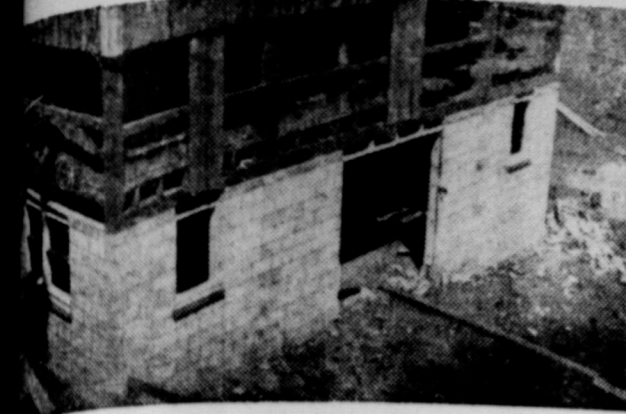
It was jacked up while a new concrete block foundation was poured for it. Then the structure was lowered to let the sills fall accurately in place on the foundation walls.
