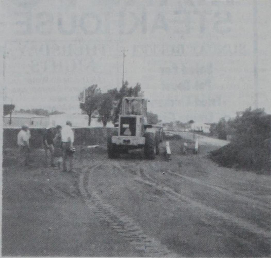
NEW SCOREBOARD TO BE ERECTED: Work is underway at Nicholson Field to get the new Scoreboard in place. Trees had to be removed and the fence at the north end of the field had to be removed. Dirt work is being done by the county to raise the grade level with the football field before the scoreboard is put into place.
