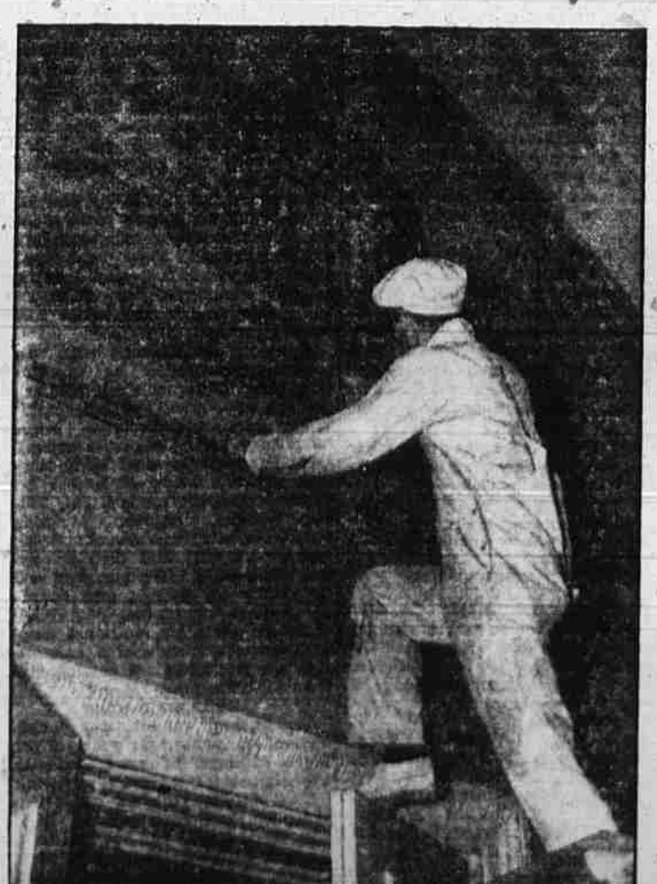
...COMPLETING THE SETTING for what may prove an historic meeting of American legislators, this painter adds the final touch to the great seal. Others replace carpets, repair furniture, scrub and paint, while still others will install an air conditioning system.
