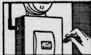
Locate the main cut-off switch at your meter box, and standing on a dry surface, turn off the electricity.
