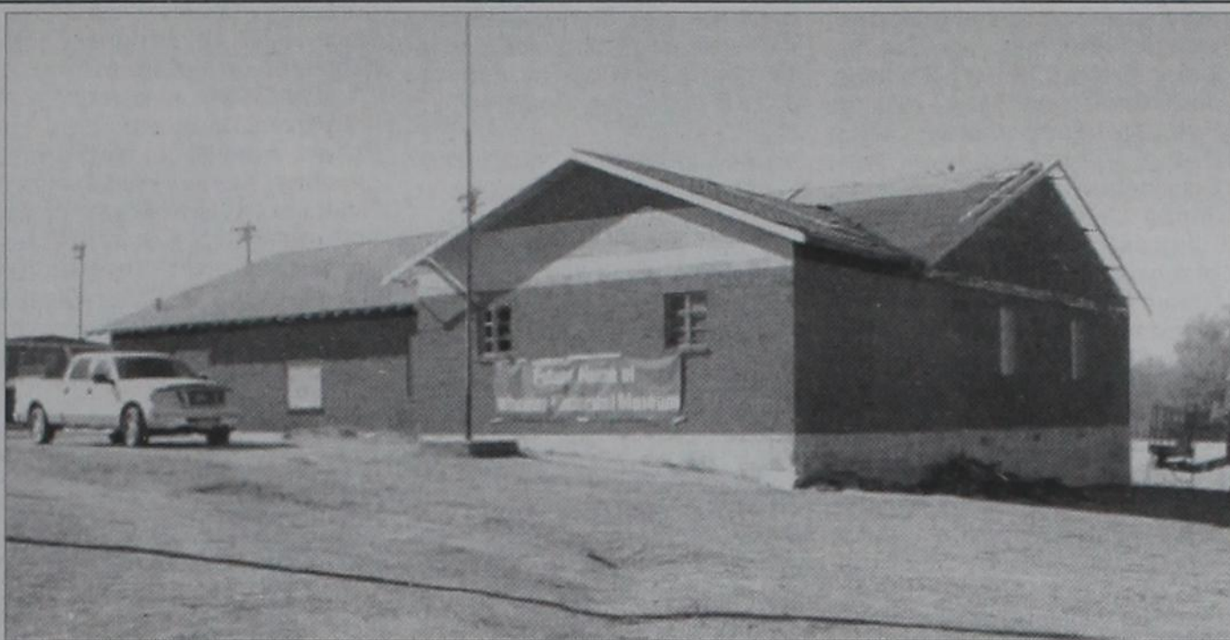
WORK BEGINS: Repair work has begun on the old American Legion building, the future home of the Wheeler Historical Museum. The first step in restoring the building is repairing the roof.
