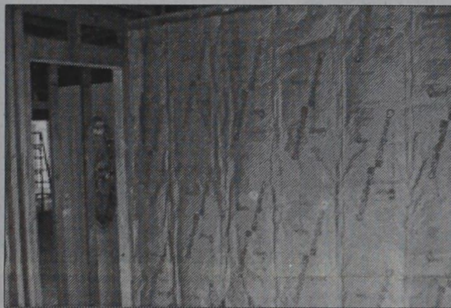
WORK CONTINUES: The interior walls of the Moore home were stripped to the studs and new insulation was also put in place.
