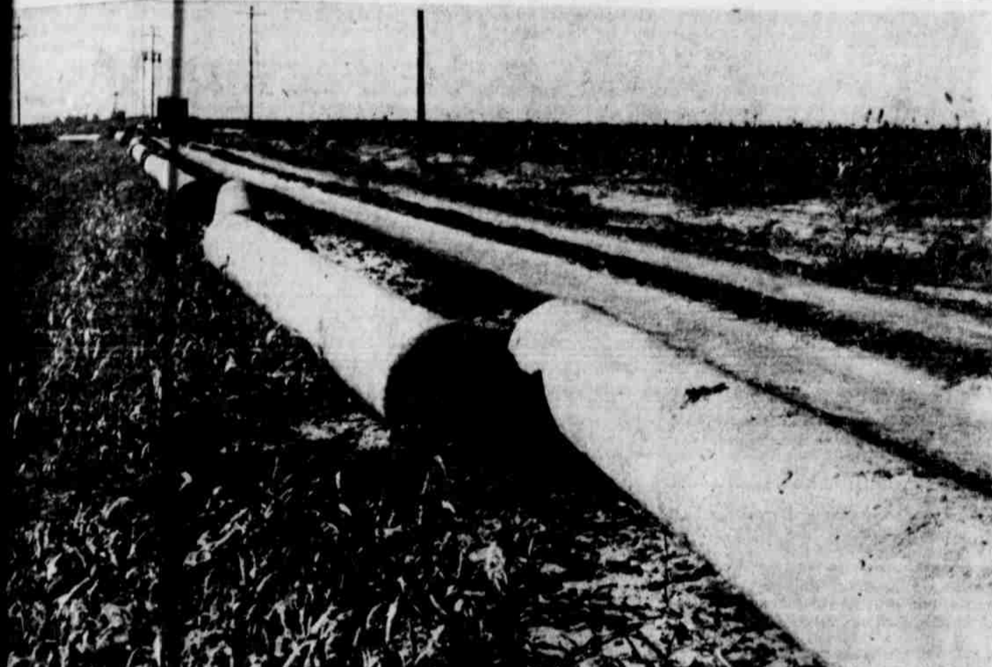
HERE'S THE PIPE for the Littlefield water works extension project. The pipe is already laid out in a string from the well house in background seen here right up to the new well sites more than a mile away. Work will begin on the project soon. (Staff Photo)
