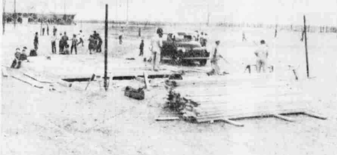
FOUR CARPENTERS employed by S. R. Duncan, Lubbock contractor, were at work at Springlake school last week building a tool house for the construction program. A week earlier employees of the contractor had surveyed and staked the foundation lines and said they planned to start digging the foundations. Meanwhile every one was expecting some sort of legal papers to be served on school officials to stop, temporarily at least, the work on the buildings.
