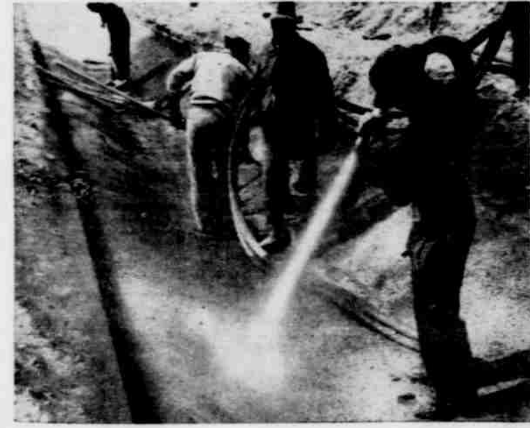
SHOTCRETE, a concrete mixture blown on with air pressure provides a smooth floor in the canals.
