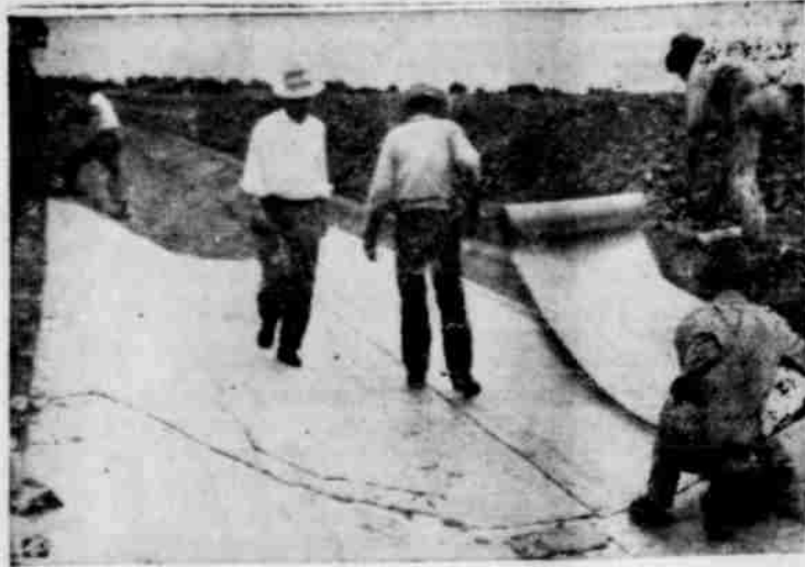
STRIPS of fiber glass are laid like carpets and an asphalt membrane is created by spraying with a hot solution.
