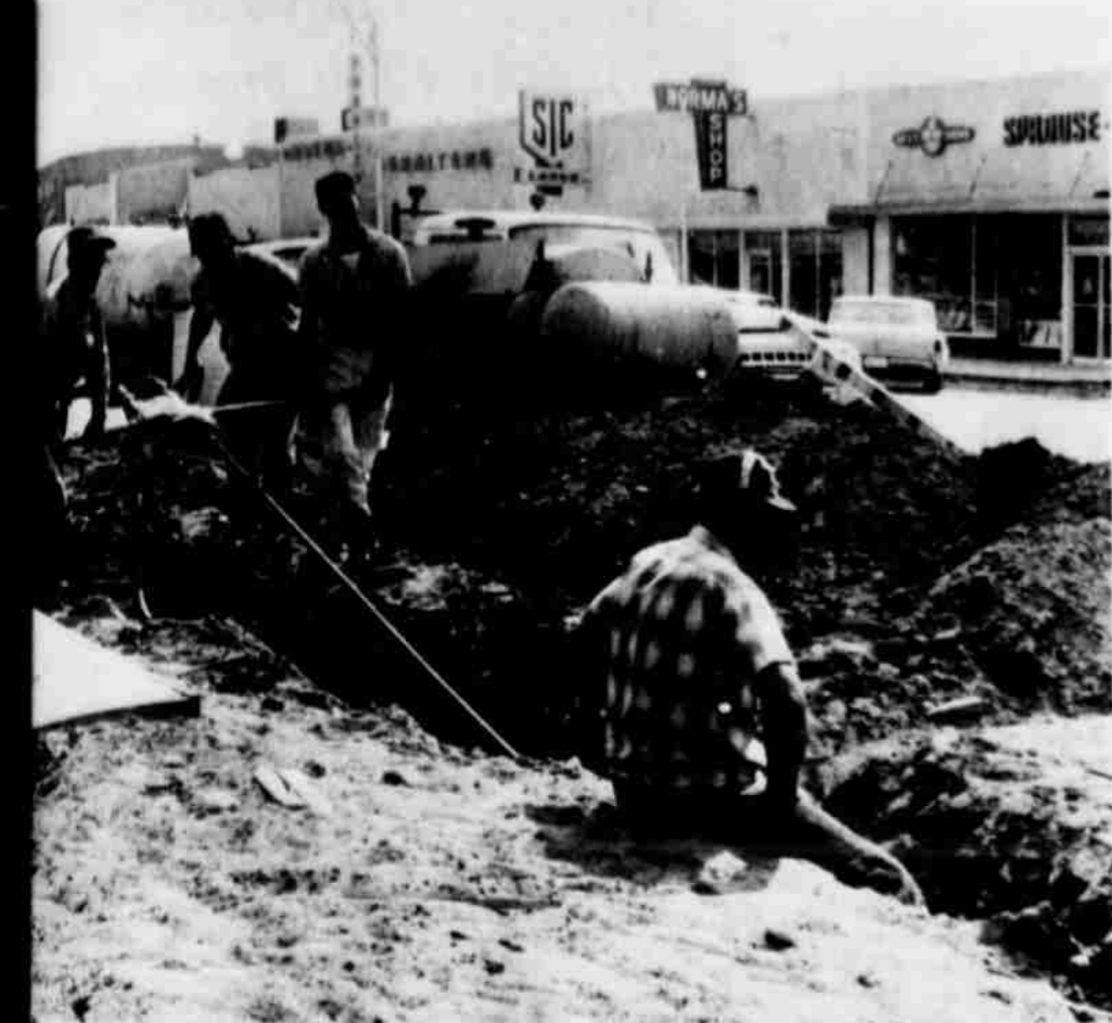
WORK GOES ON -- The Littlefield City Department has been laying new water on Phelps Ave. the past week in preparation for the crews to come back to complete
