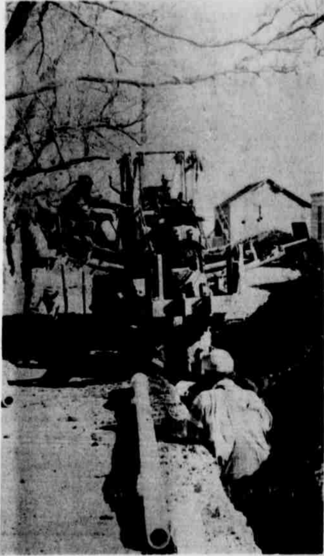
SPADE WATER LINE GOING IN--A water line can be laid quickly when a machine like this digs the ditch. Grewmen are shown laying a line for the new water distribution system at Spade. A water board was formed and a loan obtained from Farmers Home Administration for the project, which will soon provide running water for Spade community residents.
