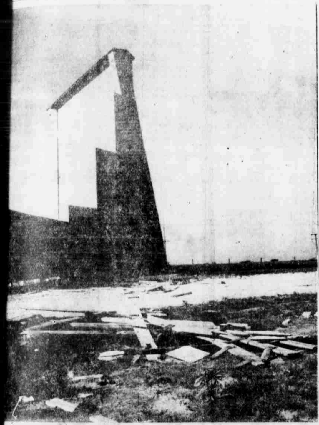
MEMORIAL DAY STORM DAMAGE is seen in this shot of the XIT Drive in theatre on the Leeland highway. The wreckage in the foreground was blown more than 100 feet by winds making a force of 70 miles per hour. The damaged portion of the screen tower, using may be seen in the dark section in the background. Showing at the XIT when the damage occurred. (Staff Photo)
