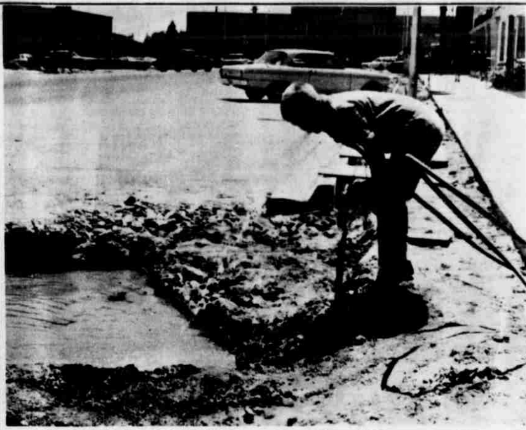
MAKING GOOD USE OF THE WATER -- When construction crews ran water into the cement laid in the crosswalk on Phelps to keep it from cracking, Jerry Cox, son of Mr. and Mrs. Bill Cox, 617 N. Sunset decided that with the temperatures in the high nineties a big drink of cool running water was just too good a thing to pass up.
