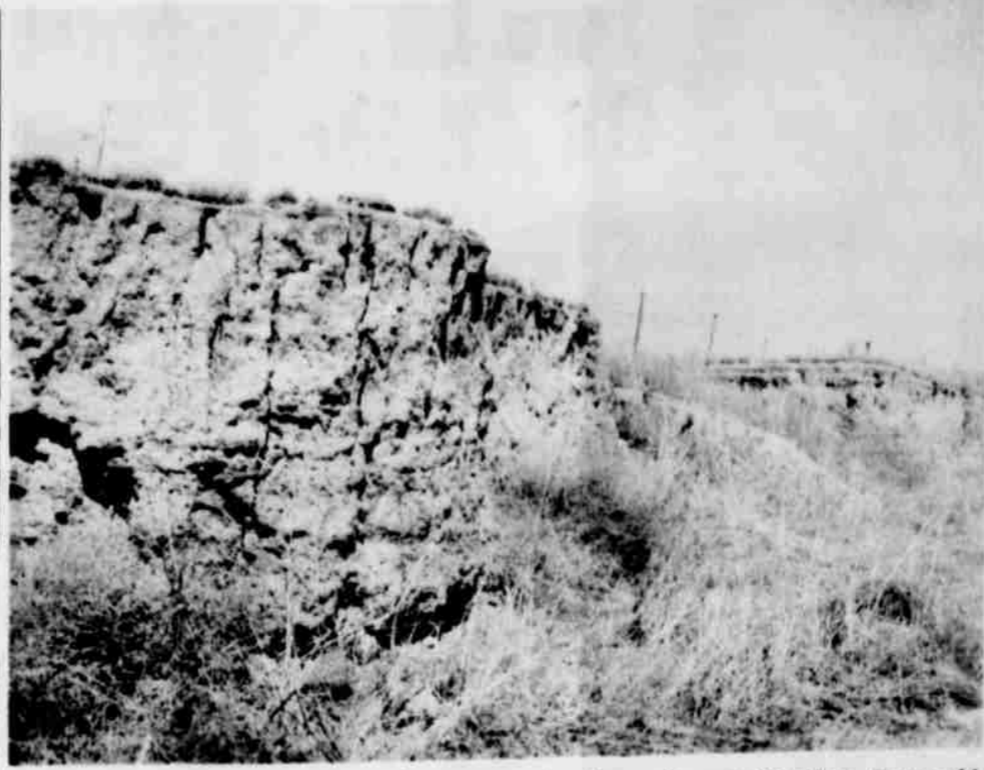
NO CONSERVATION HERE--The result of water erosion in a bar ditch is clearly illustrated in this Lamb County Soil Conservation District photo. The scene was made two miles south and two miles east of Fieldton. This could have been prevented with stabilizing conservation practices.
