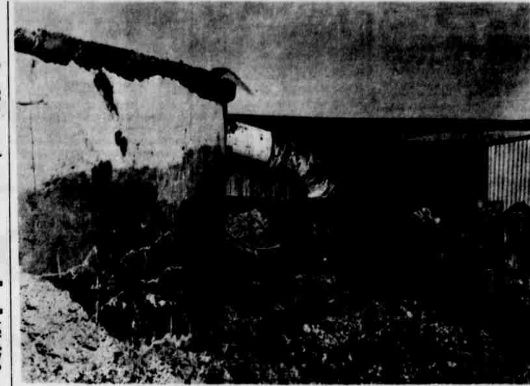
DIGGING OUT FOR REPAIRS -- Workmen are uncovering a city cement ground storage tank on Houston Ave. in order to repair cracks in the water reservoir. This is the final step in making the city eligible for a state-approved system. A 14-inch line will be installed at the same time, providing for a larger outlet into the city pumping station. The concrete tank at the Davis booster station east of town is also to be patched up. ---LEADER STAFF PHOTO
