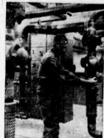
M/Sgt Davis M. Van Nortwick, Artillery, at a check point in the cooling system of the Zeus Acquisition Radar Transmitter Building. A former instructor on the Army's Nike Ajax system at Fort Bliss, Texas, Sgt Van Nortwick expects to be instructing on the ZEUS system in the near future. Home town: Robersonville, N. C.
