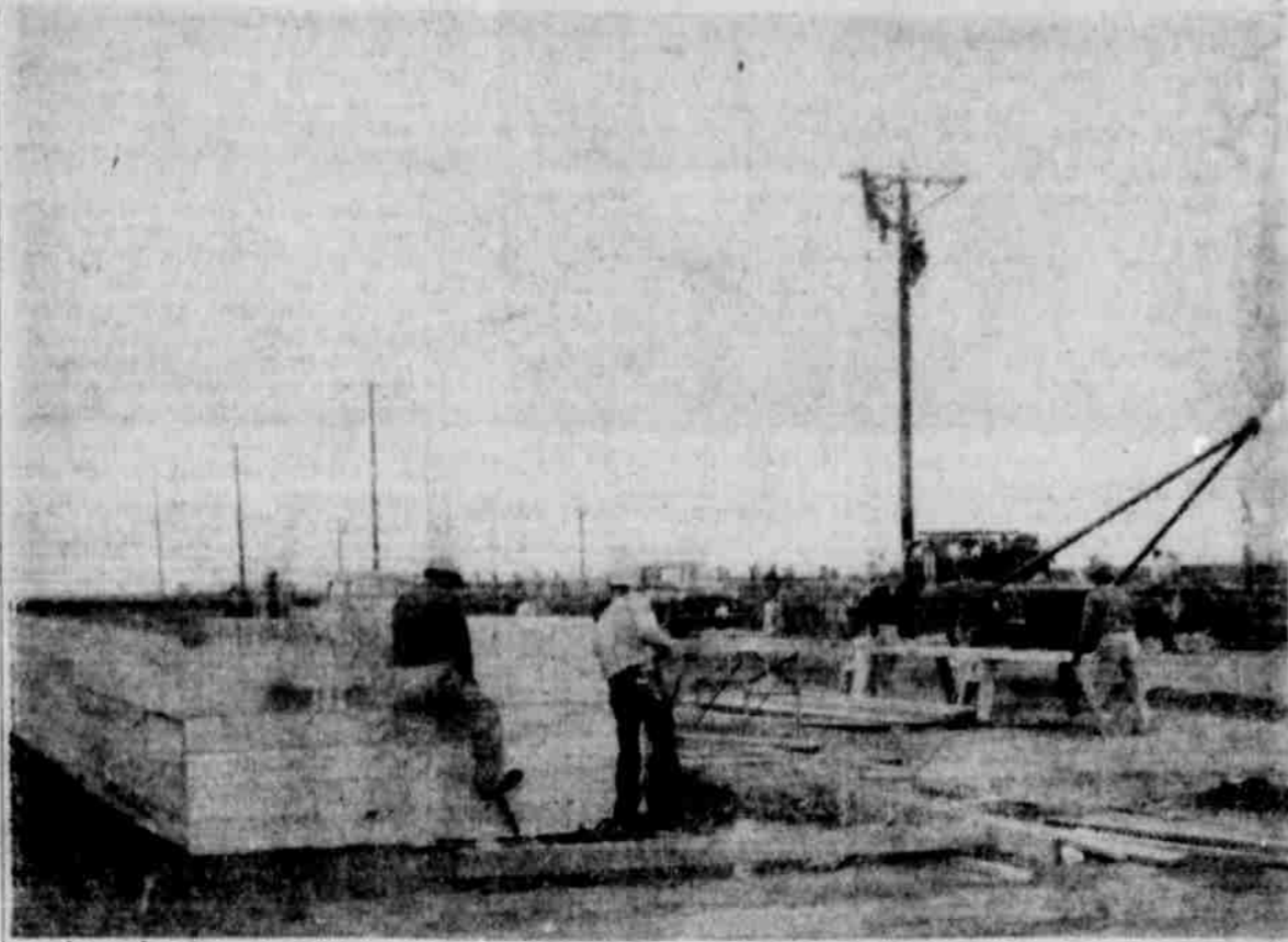
CONSTRUCTION UNDER WAY —Workers were busy early this week with the first stages of construction at the plant site of Littlefield's newest industry, the Caprock Fertilizer Co. Southwestern Public Service employees are shown setting up power at the site while men in the foreground work on a railroad loading dock. (STAFF PHOTO)
