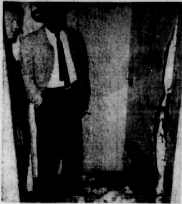
EARL RODGERS , president of the Board of Education, and Sidney Hopping, business manager for the schools, examine the more than $750 damage to the door of the vault of Littlefield High School, which occurred during Sunday night's burglary.
