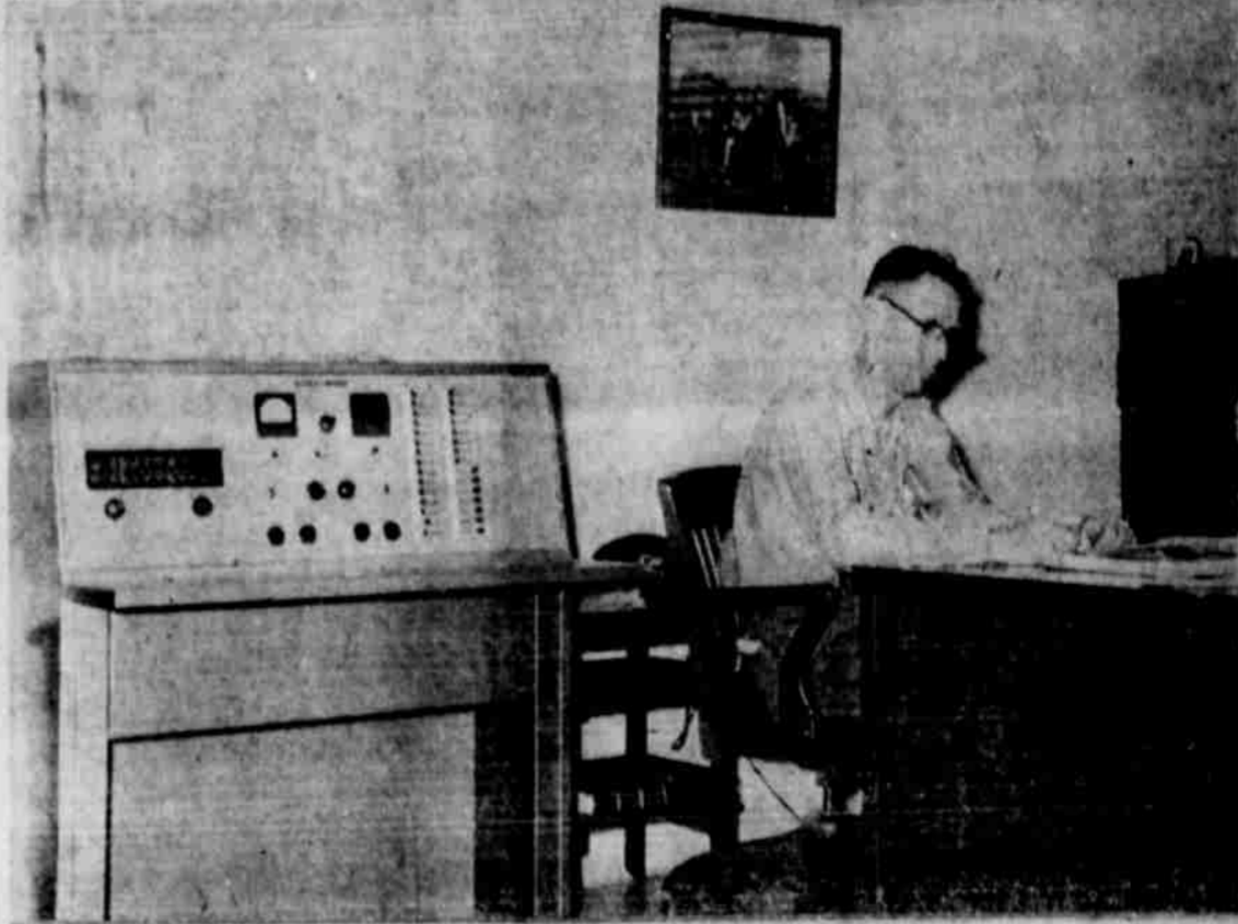
Having lots of fun learning the controls of the inter-com system has been grade school principal, Bernard Wilson. The control cabinet is located in his office and connects with all the rooms of the new Sudan building.
