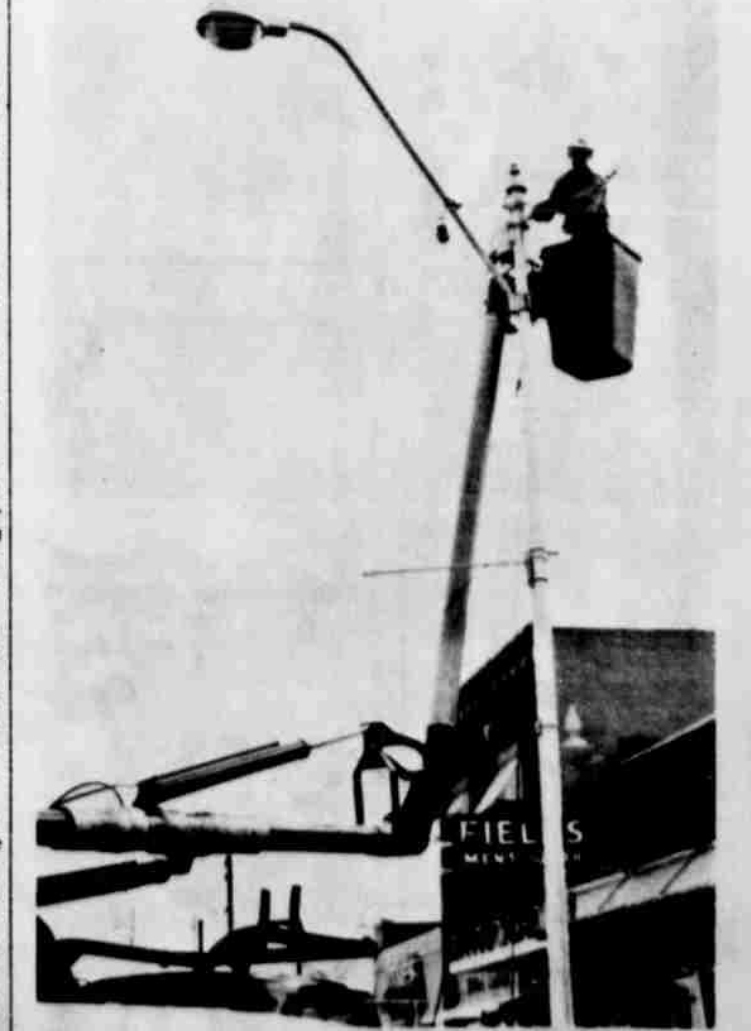
HIGH UP IN THE AIR -- The last of the overhead wires on Phelps Ave. are going down as Southwestern Public Service employees were busy at work this week cutting the overhead wires on the east side of Phelps Ave. Most of the new lights have been installed on the west side of the main street and the new poles will go up on the east side within the near future.
