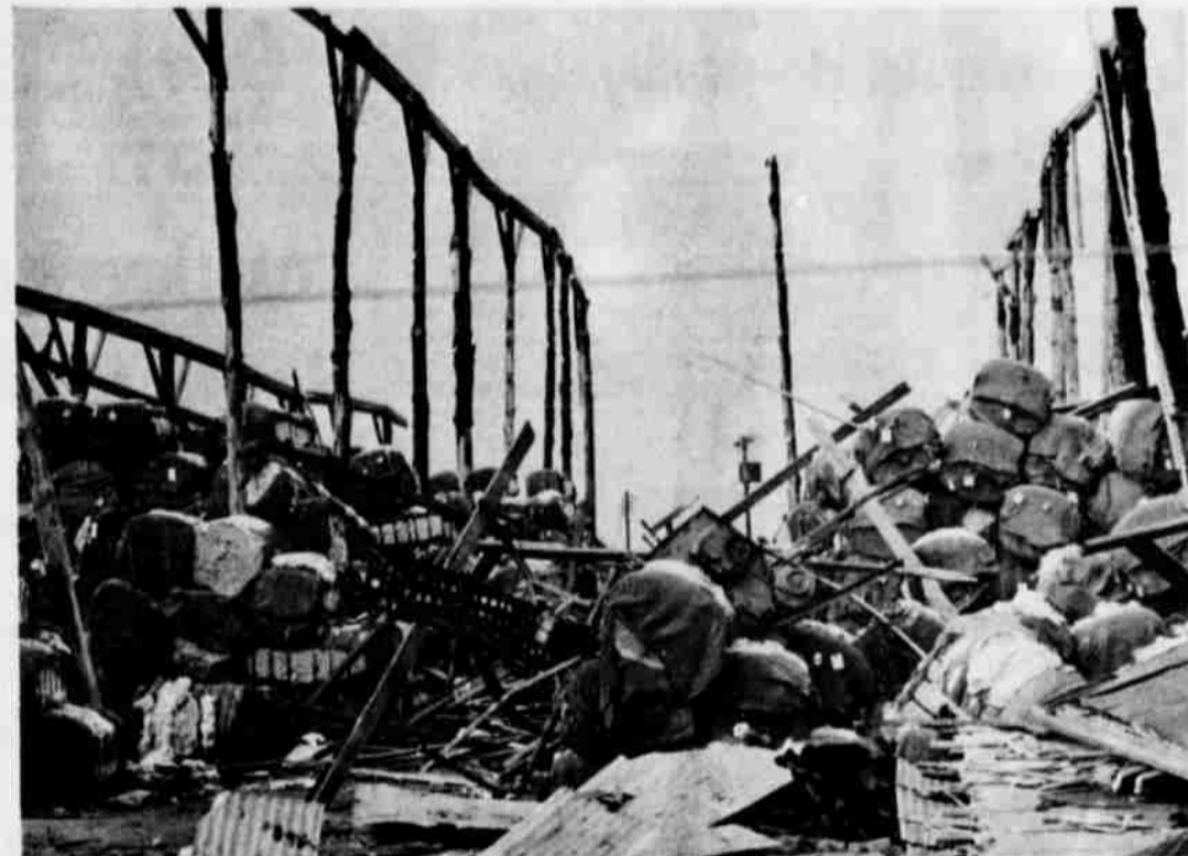
BALES OF COTTON were left exposed to hail, rain and wind when a tornado type storm transformed a warehouse of a com-
