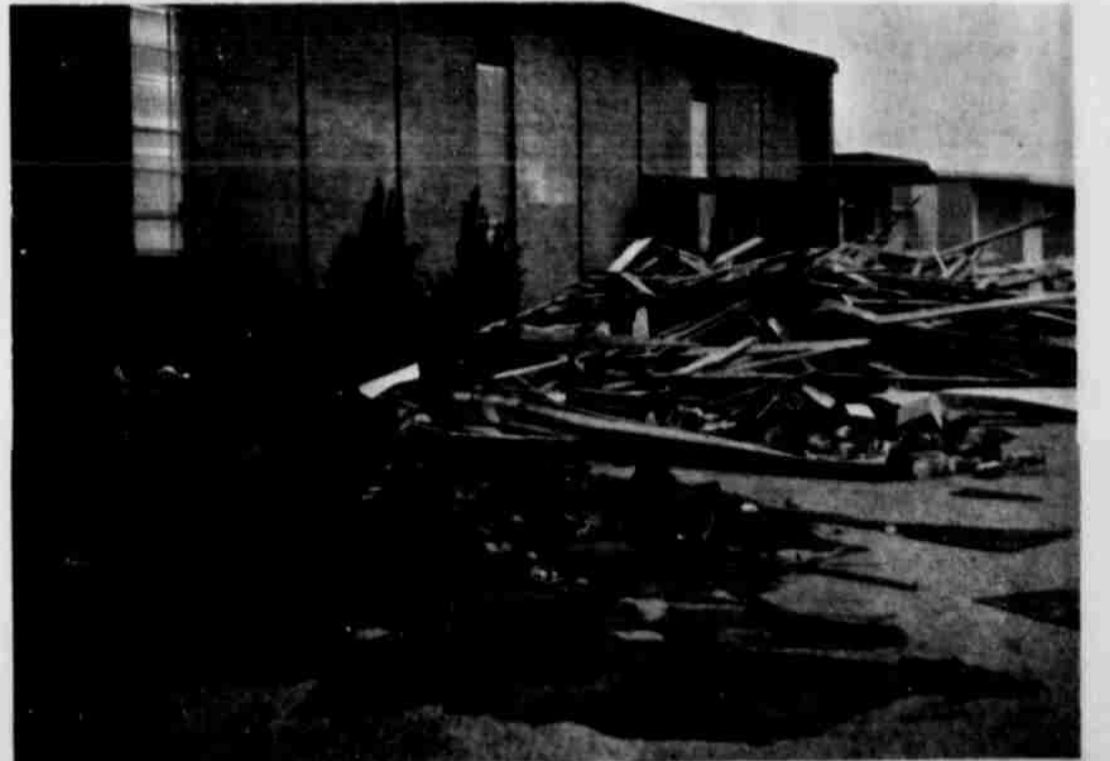
WRECKAGE is shown strewn across a portion of Springlake-Earth School grounds near the gymnasium (not shown) which lost much of its roof and sustained interior damage in Sunday night's tornadic wind and hail storm which
