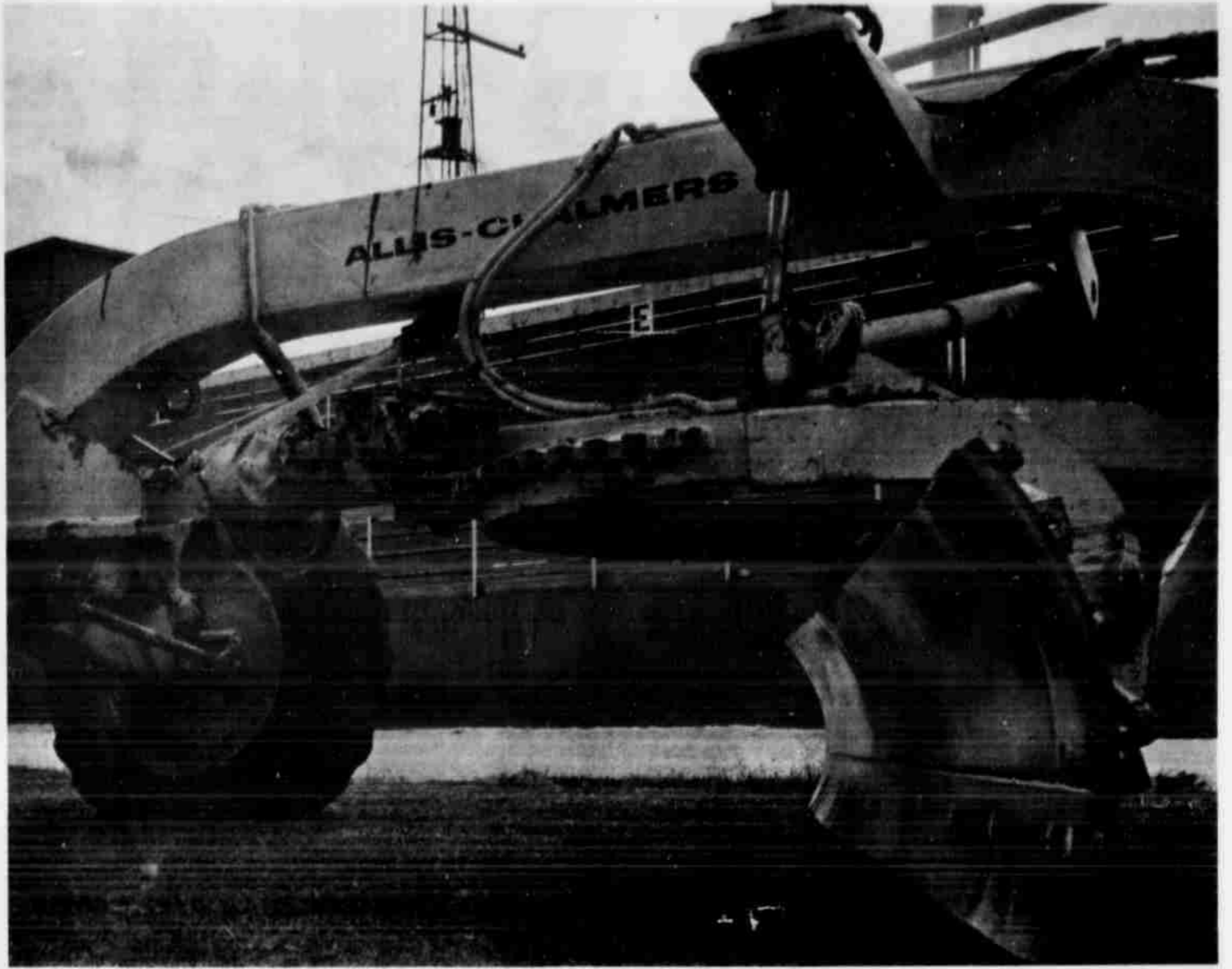
WORK IS PROGRESSING on the new track being built around the Littlefield High football field. Workmen are leveling a fine clay-rock bedding which will be used for one or two
