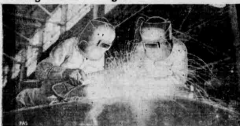
LA GRANGE, Ill. . . . These workers are welding the chassis of a diesel locomotive for the Atlantic Coast Line Railroad which placed the largest order of Diesel-electric locomotives in history. Eighteen engines will roll down the track before the job is finished.
