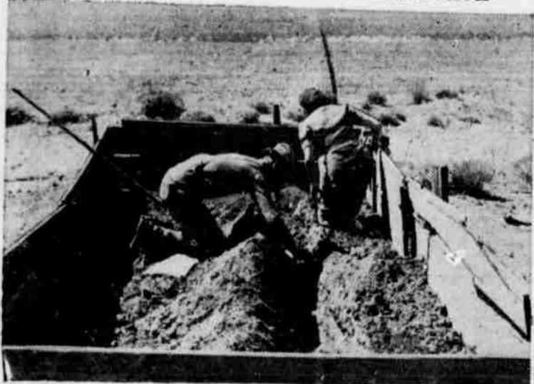
The above picture shows a frame garden under construction and old tin cans being used for the sub-irrigation. An outstanding feature of these frame gardens is the fact that fresh vegetables can be grown for the family tables long before the ordinary gardens are in production, and for many weeks after the first frost in the fall. An ordinary sized frame garden will produce all an average family needs for daily use.
