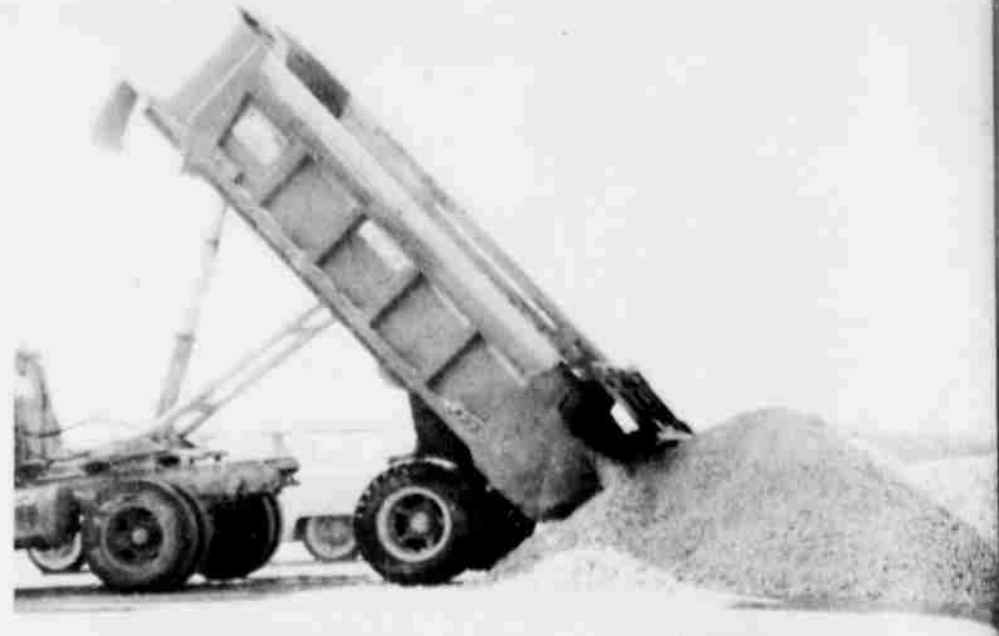
BEWARE OF TRUCKS ON 84 -- Large gravel trucks are running constantly now on Highway 84 southeast of Littlefield in the area where the road is being constructed. Highway officials warn motorists to be on the lookout for the trucks and continue to drive carefully in the area under construction.
