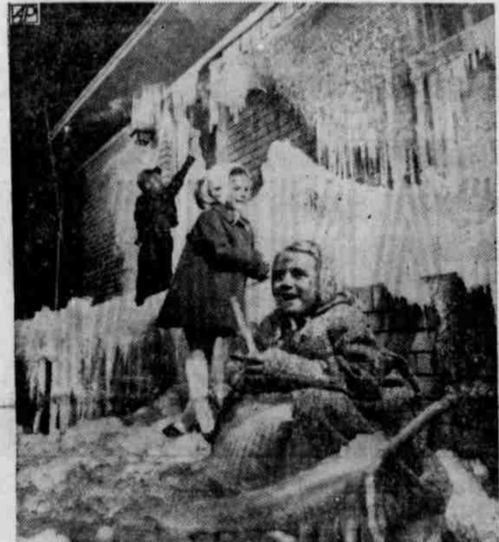
RESULT OF ICY NORTHER —The norther which struck across Texas left this broken pipe and icy house in Dallas. When expanding ice broke the pipe it sprayed water, which quickly froze, over the unoccupied house. The children are, front to back: Kathy Shuhart, 7; Pamela Remaley, 6, and Gary Shuhart, 5. (AP PHOTO)
