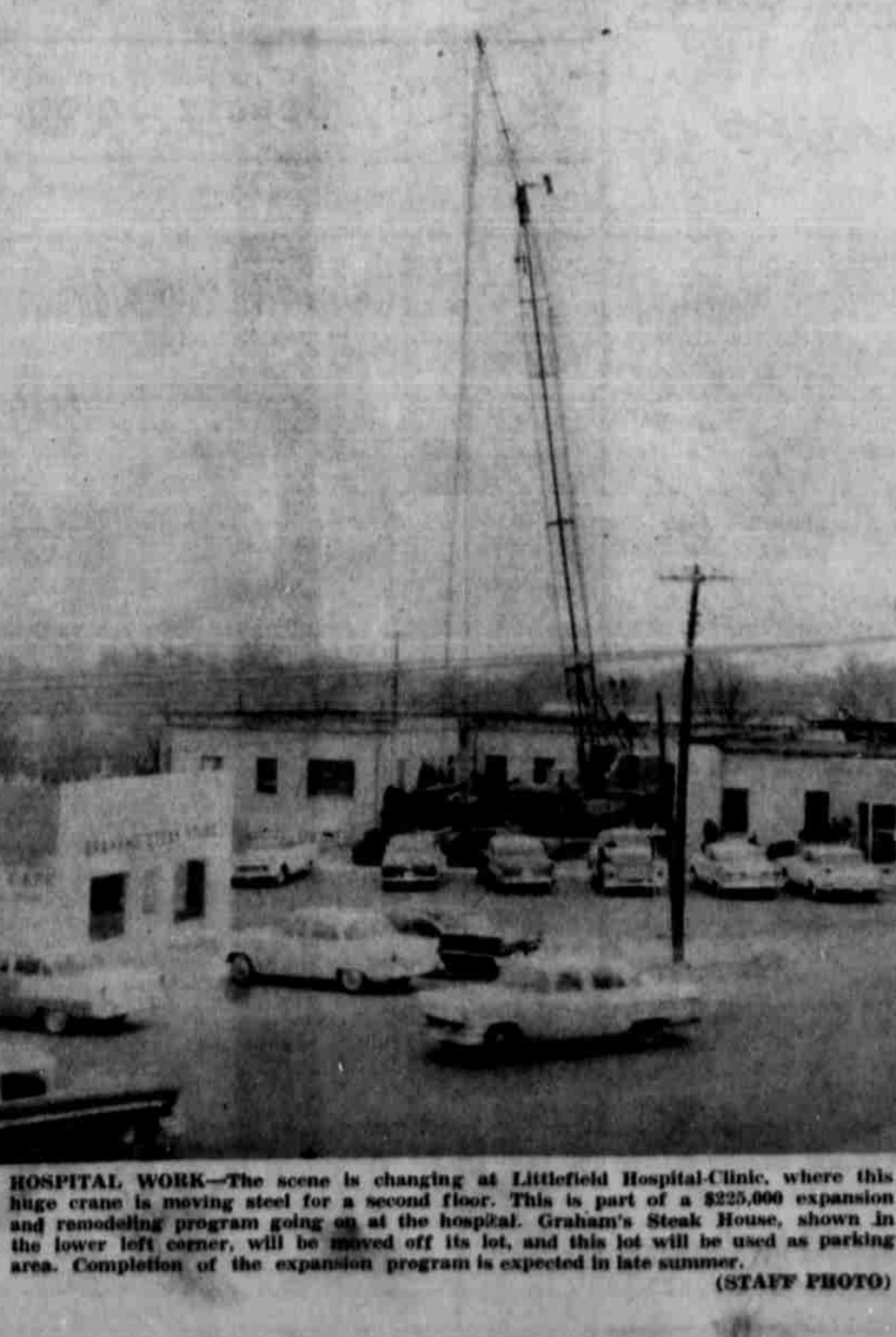
HOSPITAL WORK—The scene is changing at Littlefield Hospital-Clinic, where this huge crane is moving steel for a second floor. This is part of a $225,000 expansion and remodeling program going on at the hospital. Graham's Steak House, shown in the lower left corner, will be moved off its lot, and this lot will be used as parking area. Completion of the expansion program is expected in late summer. (STAFF PHOTO)
