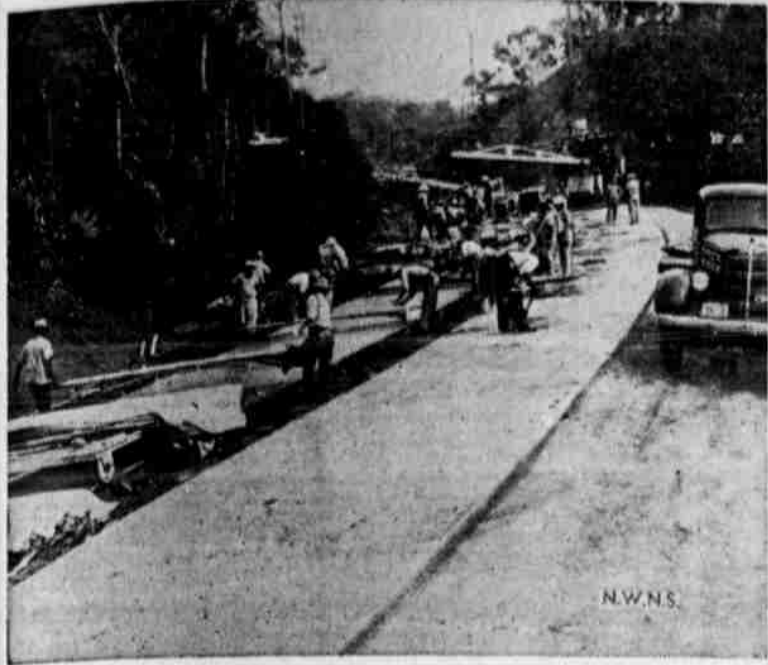
Concrete crews in the Canal Zone are shown at work on a section of the new Trans-Isthmian highway that Uncle Sam is building, at top speed across the Isthmus of Panama, to link the ocean terminals of the vital canal. The new highway will enable defense forces to move from one end to the other in two hours. Big rush of the moment is to beat the coming of the rainy season.
