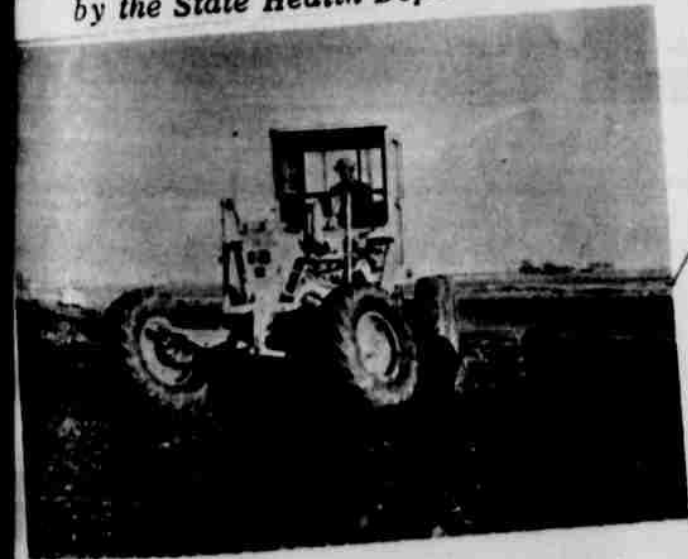
... 1964 marked the beginning of work on the $810,000 Highway 84 by-pass that will lead to future growth of the community.
