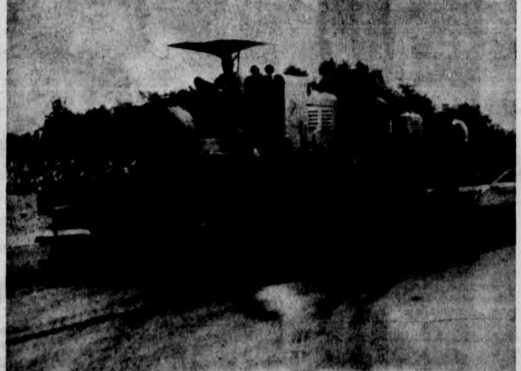
PAVING SPEEDED —The big machine above is making quick work of Littlefield's 87-block paving program as final topping is applied. The machine above was winding up the topping procedure on Sunset, a 22-block project and the longest single paving strip in the program. (STAFF PHOTO)
